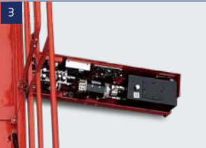
Hydraulic and electric system
